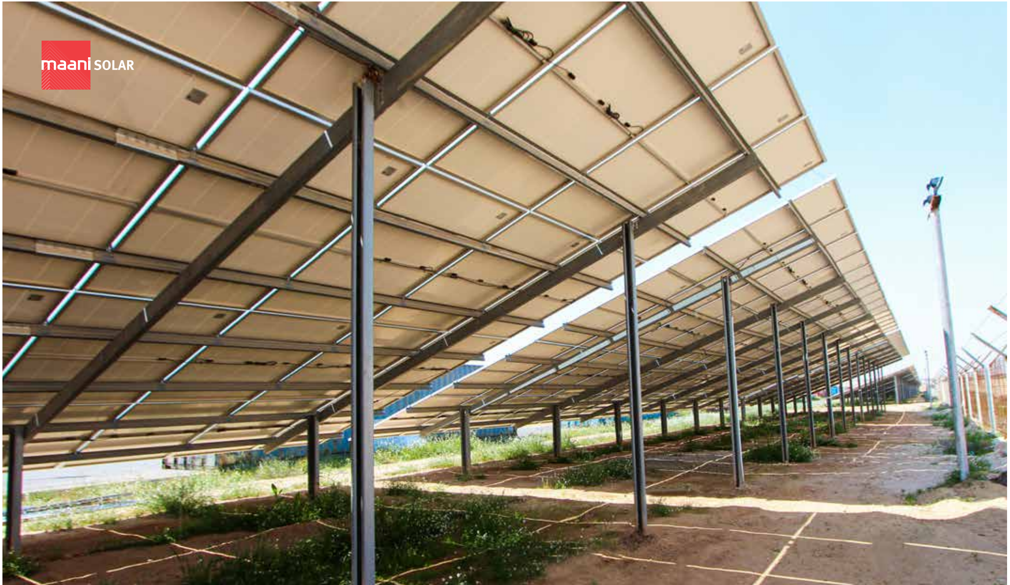
Title: JADARA Equipment & Defense Systems Co. Location: Zarqa, Jordan Scope: On-grid photovoltaic 712 kWp / 600 kWac system
